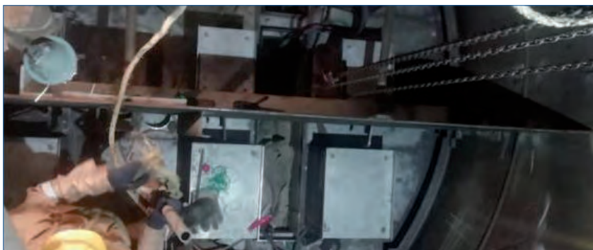
Figure 3B Dividing wall being installed during a revamp of a conventional column in South East Asia (Image courtesy of DWC Innovations)
