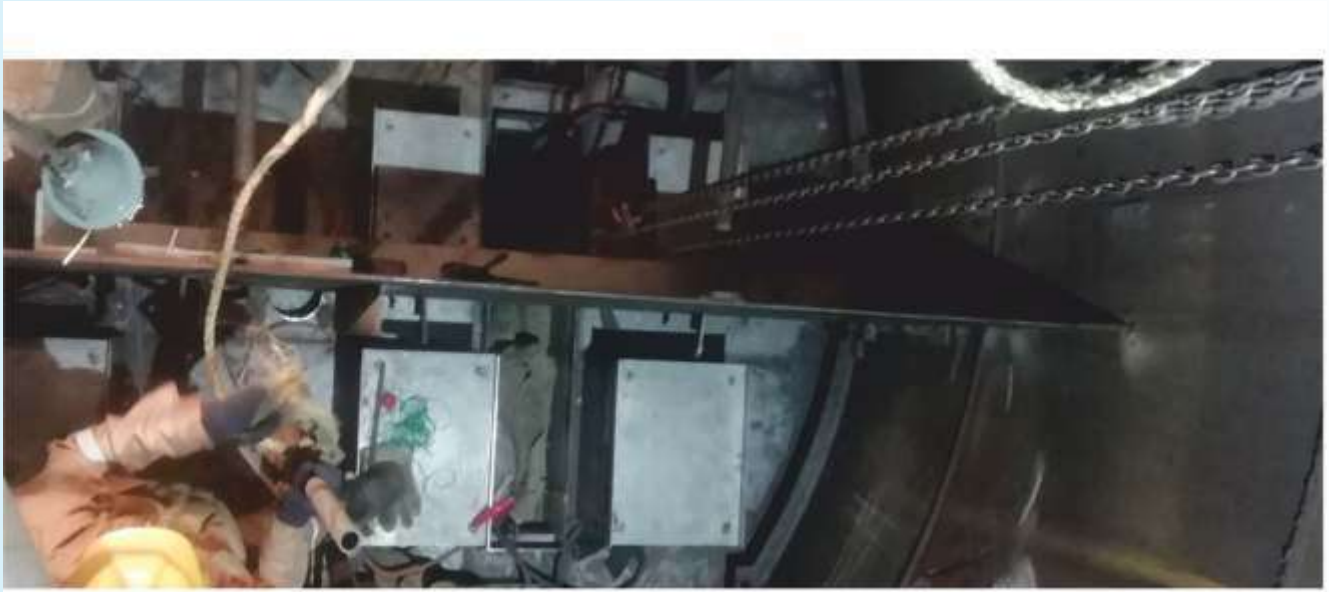
Figure 3B : Dividing wall being installed during a revamp of a conventional column in South East Asia. (Image courtesy of DWC Innovations)
